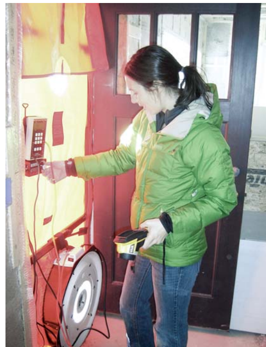
Figure 8. Blower-door testing at the weathertight stage is effective for early detection and treatment of air leaks in the envelope. The author achieved remarkable levels for this stage of construction.
