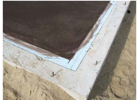
Figure 1. Four-inch-thick foam board provides R-20 insulation under and around the edges of the radiant floor slab (left), which is tinted chocolate brown to serve as the finished floor. The inside 2x4 wall of the 11 1 / 4 -inch-thick double framing will cover the exposed foam around the perimeter (above).
