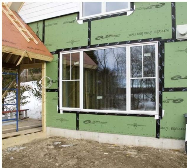
Figure 3. Triple-glazed windows cost up to 50 percent more than comparable double-glazed units but — according to computer modeling — will represent a 20 percent gain over double-pane glazing in the building's energy performance.
