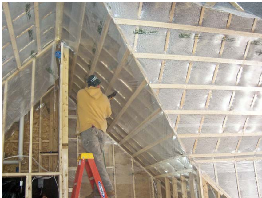
Figure 9. Triple-ply Par/Pac membrane is stretched around framing edges and rigorously stapled to prevent the cellulose insulation from bulging past the wall plane. Cellulose is blown through slits in the membrane to a density of 3.5 pounds per cubic foot. The slits are then resealed with tape.
